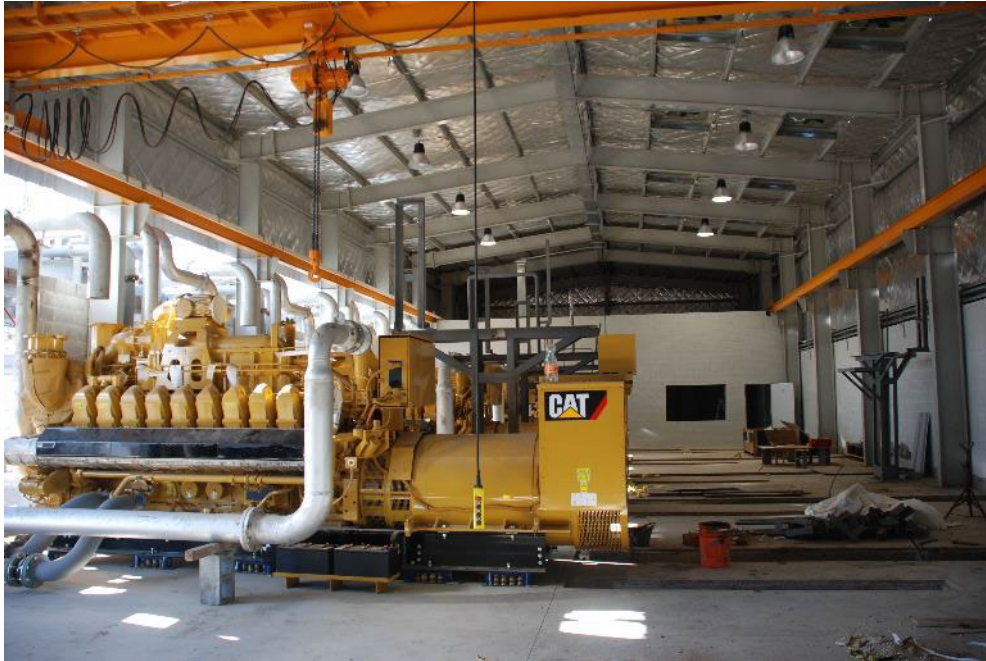
1 GENREM CONTRACT SAN MIGUEL NIIC 10 Mwh
